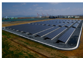
The solar power plant that supplies electricity to Hibikinada Greenfarm
