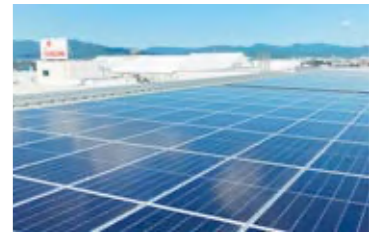
Solar panels at the Kozakai Plant
