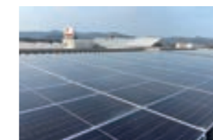
We have installed solar panels at the Kozakai and Ibaraki plants, which began generating electricity in April 2021.
