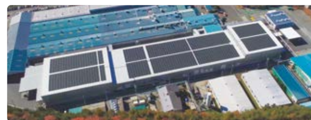
Solar panels installed at Fujimi Plant (Nagano Prefecture)
